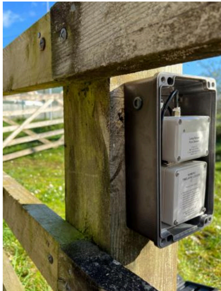
Post-mounted pyro sensor
